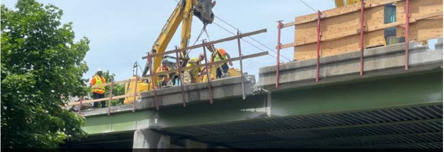
NYS DOT, Bridge Repair of NY 27 Westbound Over Barnes Road Silver Award, Transportation
