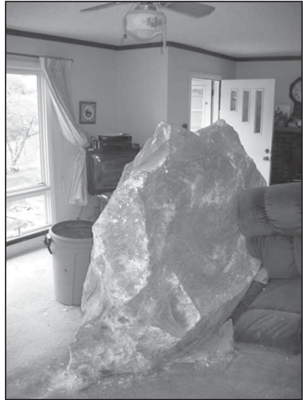
Rock in a Glenwood Springs living room, 2004. The owner of this home had built a relatively small rockfall barrier above the home. The rock entered the home from the right side of the picture. Colorado Geological Survey photo.
