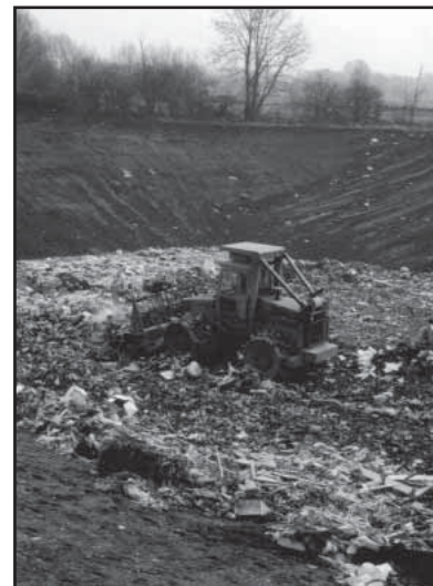
Figure 1. Industrial waste disposal in dry gravel workings with clay liner (Courtesy RMC Group).
