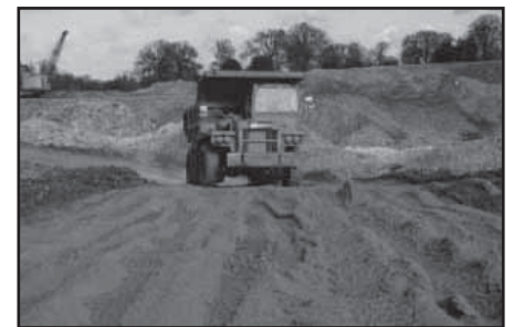
Figure 3. Drag-line excavation in glacial sands and gravels at Ware, Hertfordshire and transport by dumper truck to processing plant (Courtesy RMC Group).
