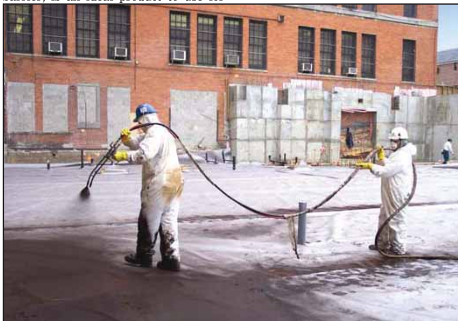
Figure 2. Installation of a fluid-applied vapor barrier at a public school in Queens, NY.
