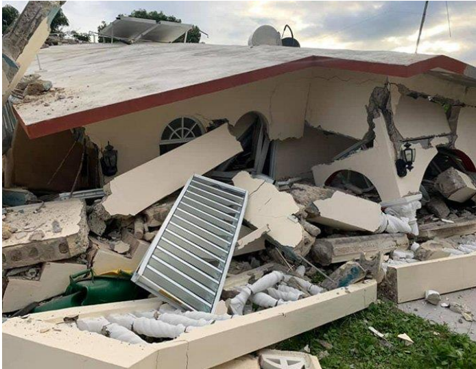
Residential earthquake damage. Guánica, Puerto Rico
