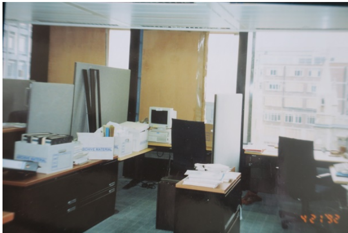
Works started quickly to repair the damage, with the empty window panes boarded up where the glass had been blown out.
