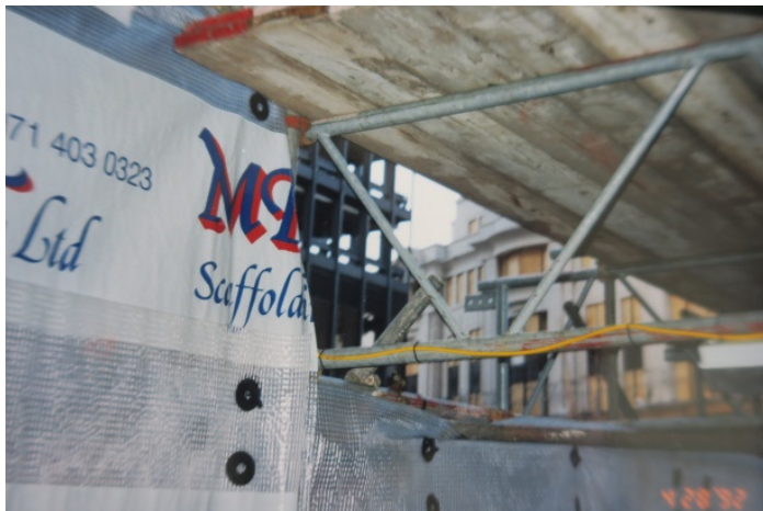
These repair works clearly limited the views from HQ, as scaffolding was put up to replace the windows.
