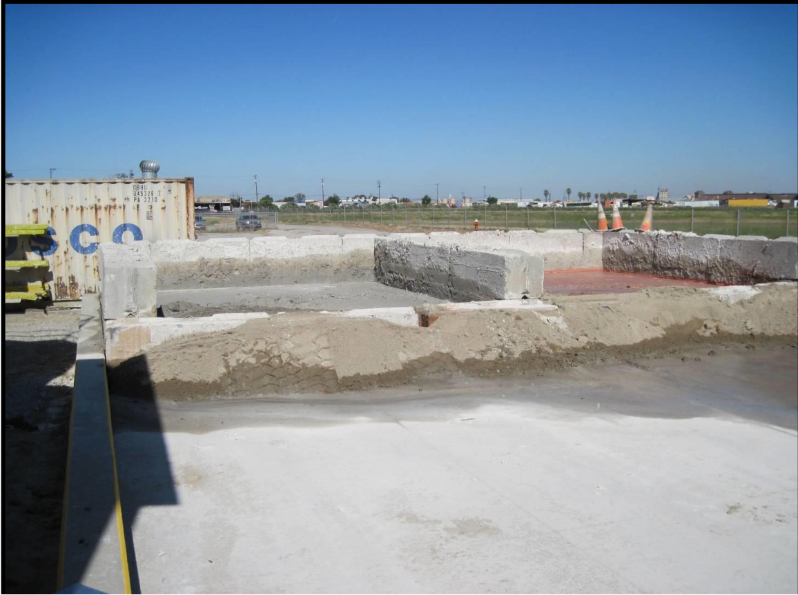
Two-bay Schmütz drying pad, one bay used for color washout only.
