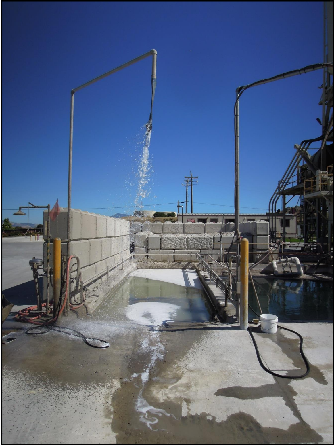
Process Water Equipment for Washout of Mixer Drum
