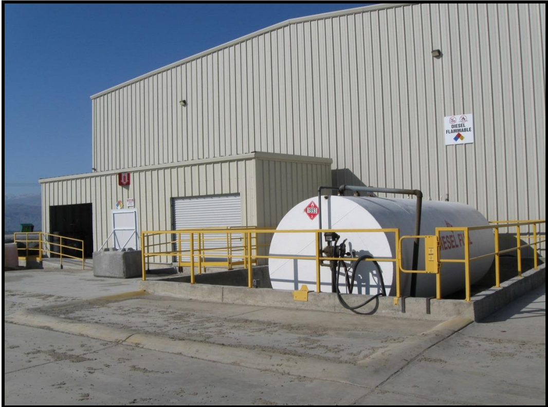
Secondary containment for hazardous materials
