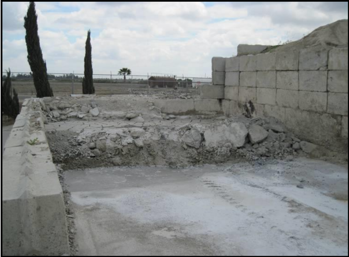
Single bay Schmütz drying pad built on a concrete pad using “Bin Blocks”
