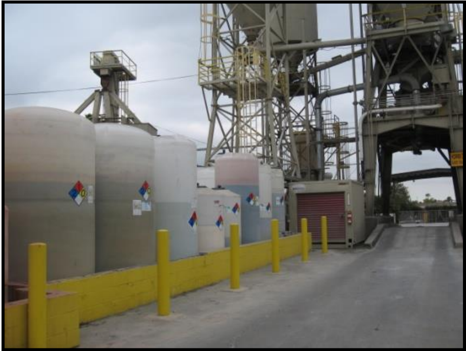
Secondary containment for Admixtures
