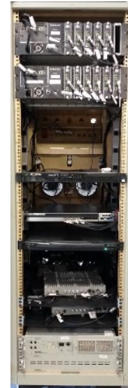
Satellite Television System (STS)
