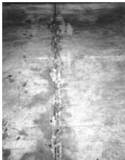
Joints damaged by solid-tyred reach trucks
