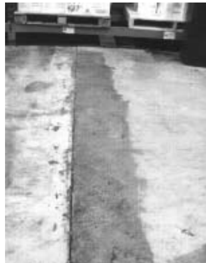
Loss of surface by abrasion
