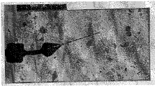
Figure 11 Plane section from Full Scale Trial Casting showing complete casting-in of waterstop [4]
