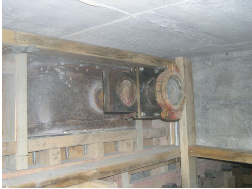
Fig 9. Pumping Valve in Position
