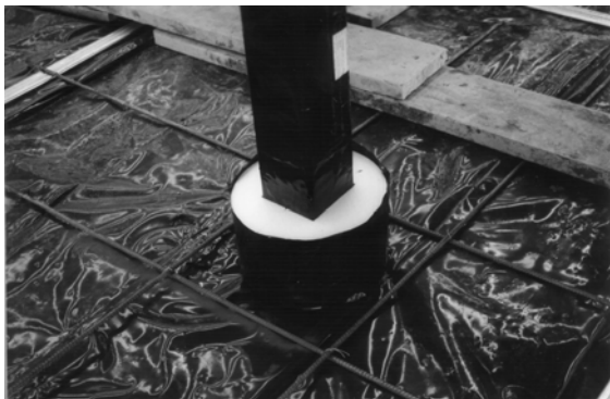
Figure 11 Slab penetrations such as portal legs are isolated using contoured polystyrene block outs. Note that the portal leg has been wrapped in polythene to protect it from concrete splash.
