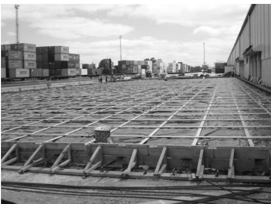
Figure 18 The external pavement is 270 mm thick. This generated a large amount of heat of hydration.
