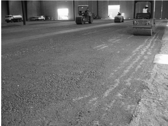
Figure 10 The sub base needed to be finished to tight tolerances to reduce the risk of the floor cracking.
