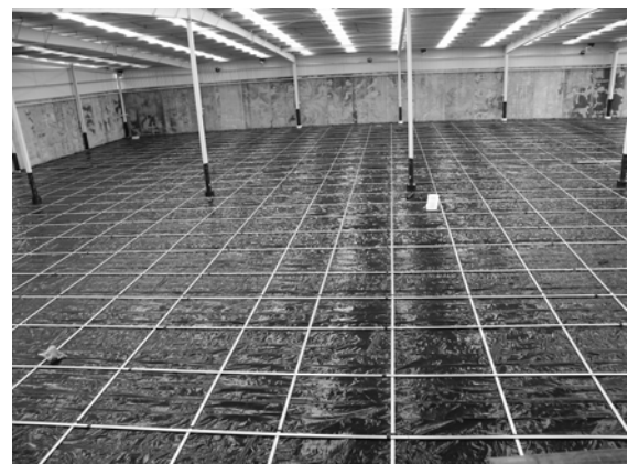
Figure 13 PT ducting makes it impractical to discharge concrete directly from trucks.
