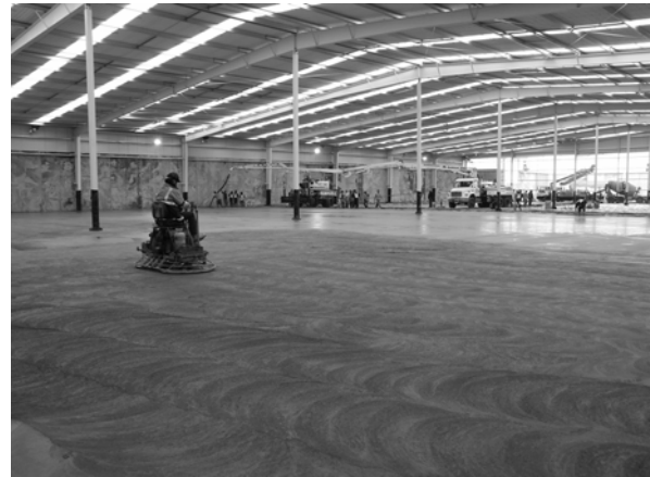
Figure 16 Finishing begins at one end of the building while concrete is still being poured at the other end.
