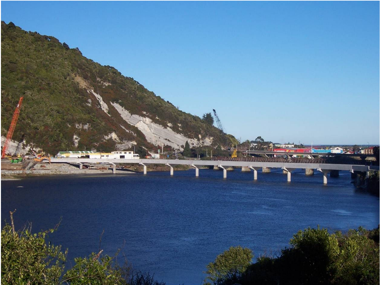
Figure 5 Completed new Bridge 1 Rapahoe before removal of the original bridge in the background
