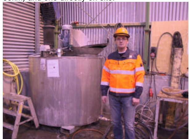
Figure 6: Mixer for the site production of the liquid alkali-free accelerator
