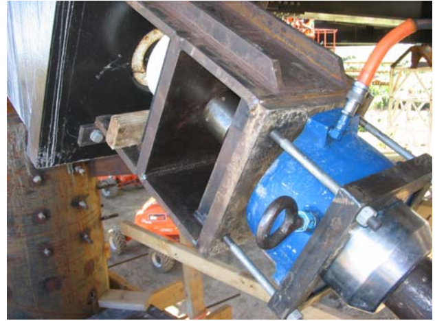
Figure 15. Stay tensioning arrangement. The 2 stage trestle allows the jack to be cycled and retain load in the stay.
