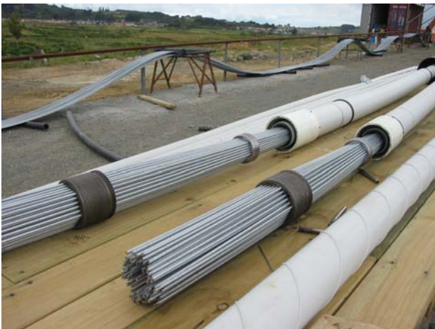
Figure 10. Wire bundles inserted in stays prior to button heading. Note cutting line and pre-cut wires in the background and turbulence inducers on the HDPE duct in foreground.
