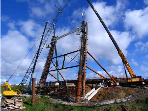
Figure 3. Erection of the steel portal beam and pylon anchorage on top of the column formers prior to pouring
