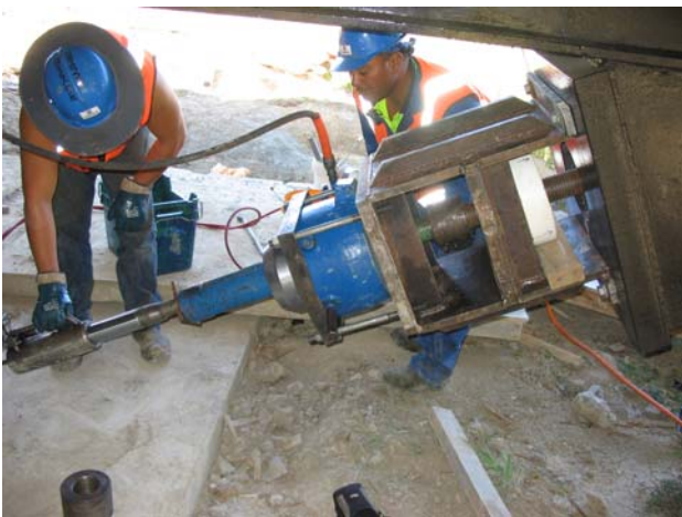
Figure 14. Stay tensioning arrangement. Note the small capacity jack being used to pull the pull rod through the large hydraulic jack.
