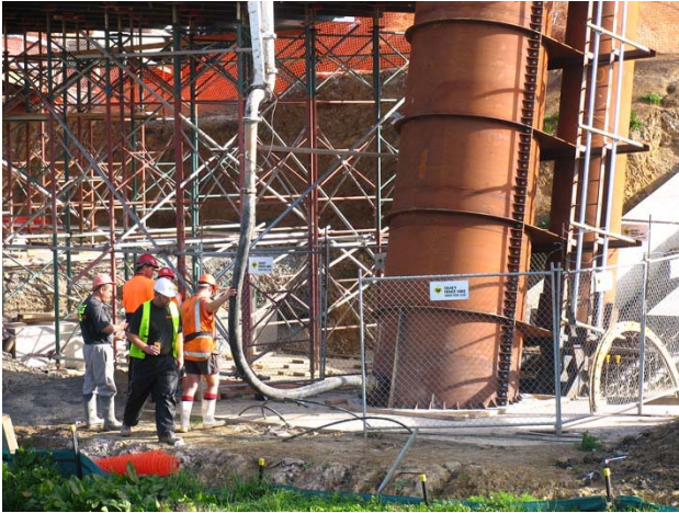
Figure 4. Base pumping self compacting concrete into the 28m high reinforced concrete pylons
