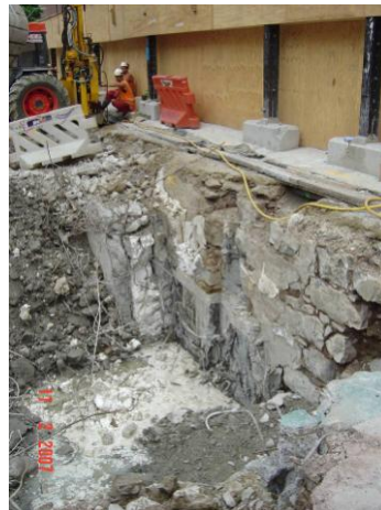
Bluestone wall obstruction
