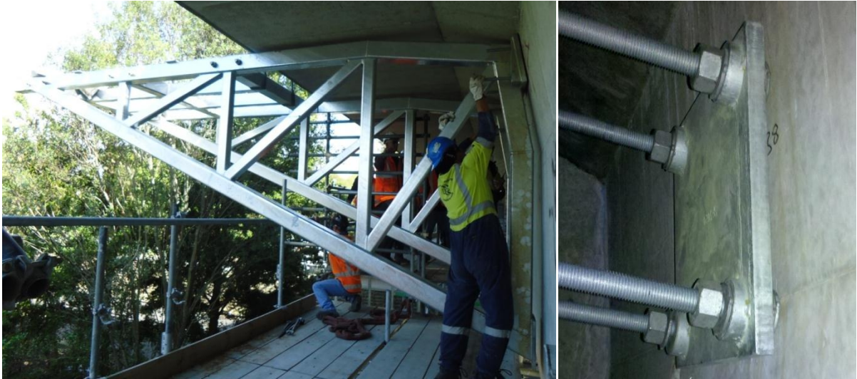
Figure 12 and 13. First frame set erection and close up of the internal upper connection
