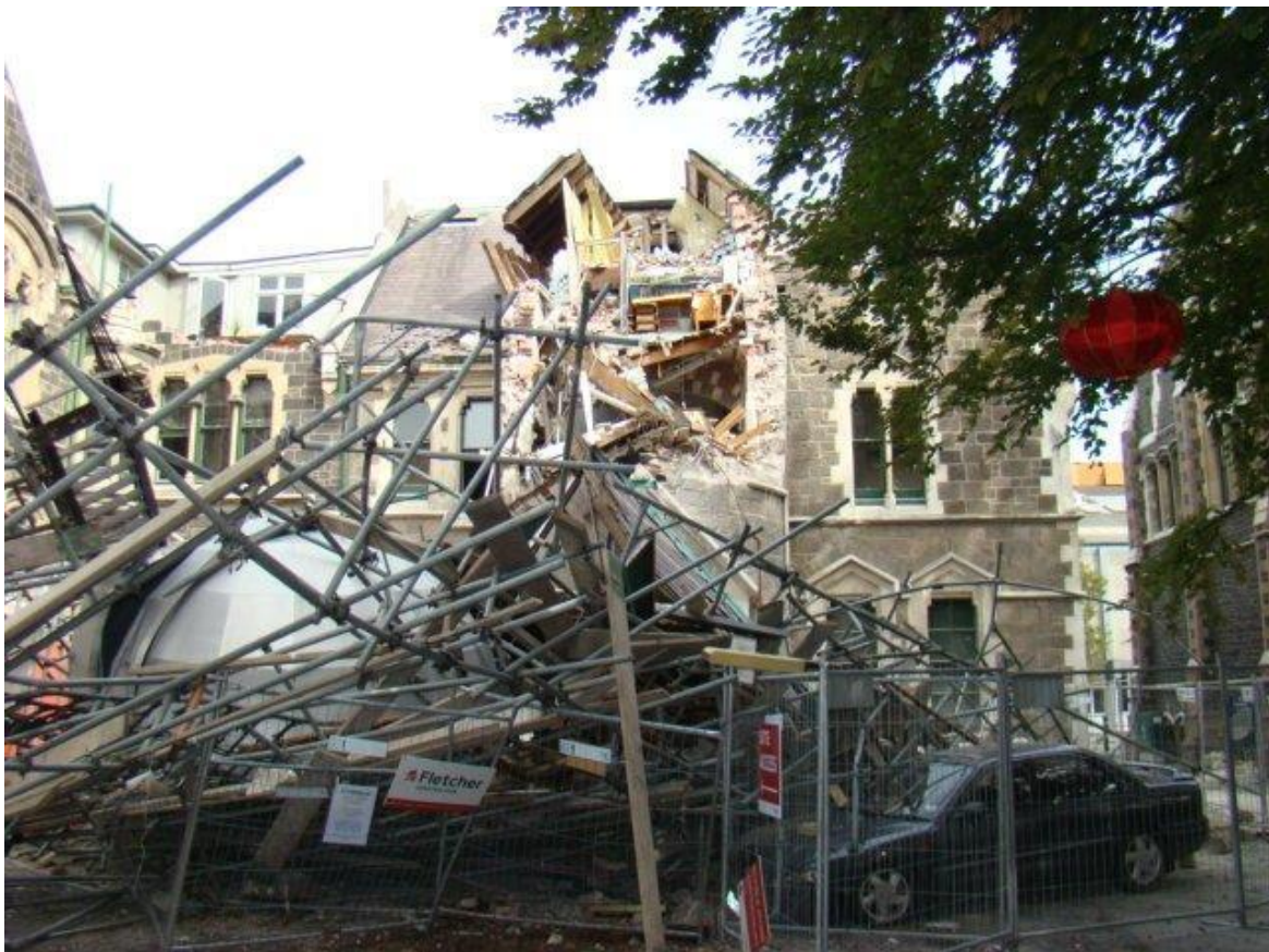
Figure 2. Photograph Showing the Damage to the Observatory Tower Incurred from the February 2011 Earthquake
