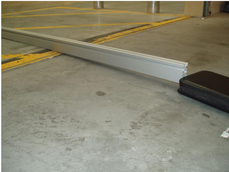
Figure 7 Slab curl in a typical New Zealand floor
