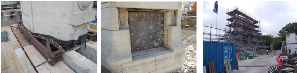
Figure 4. (L-R) Steel Column Clamp, Temporary Access Hatch in side of Column, Scaffolding
