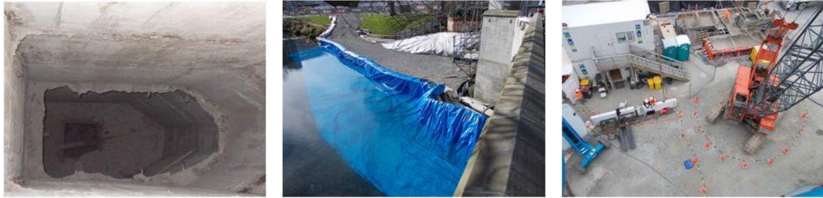
Figure 5. (L-R) Inside of Major Column, Access track and Dam, Site setup during Piling
