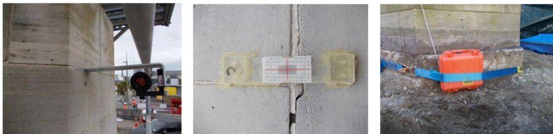
Figure 3. (L-R) Survey prism, Crack Tell-Tale visual monitor, Vibration monitoring sensor
