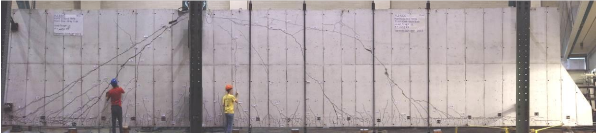
Figure 10. Specimen PLS4000 after failure of short shear span with shear reinforcement
