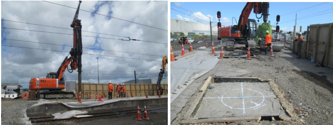
Figure 7: Piling during enable work, note the proximity to the overhead electrified lines.
