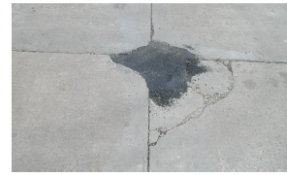
Figure 13. Corner crack-off repaired with temporary repair using asphalt
