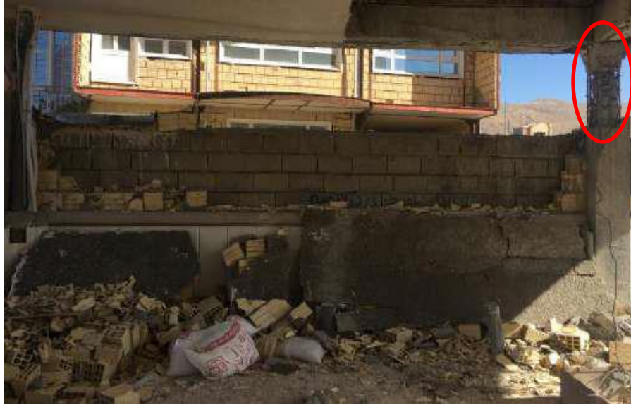
Figure 5. Short column failure due to presence of masonry infill
