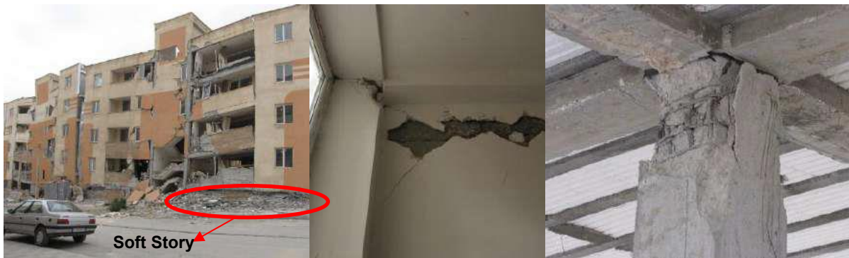
Figure 8. Shear failure in column and shear wall and soft story because of poor quality concrete.
