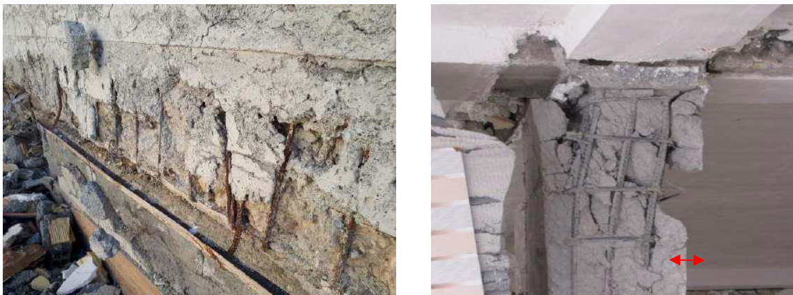
Figure 9. a) Insufficient concrete cover, b) excessive column concrete cover and spalling of concrete cover.
