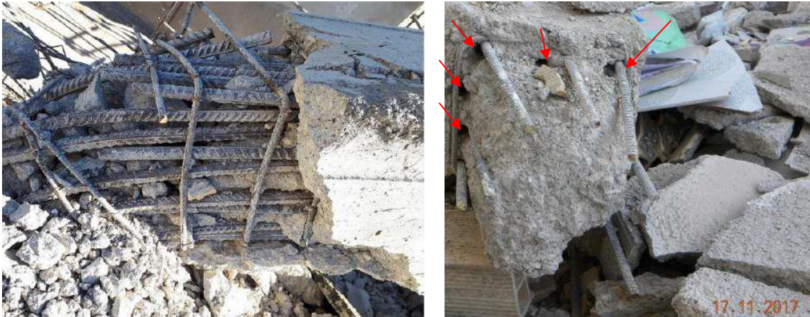
Figure 11. Insufficient lap splice in column
