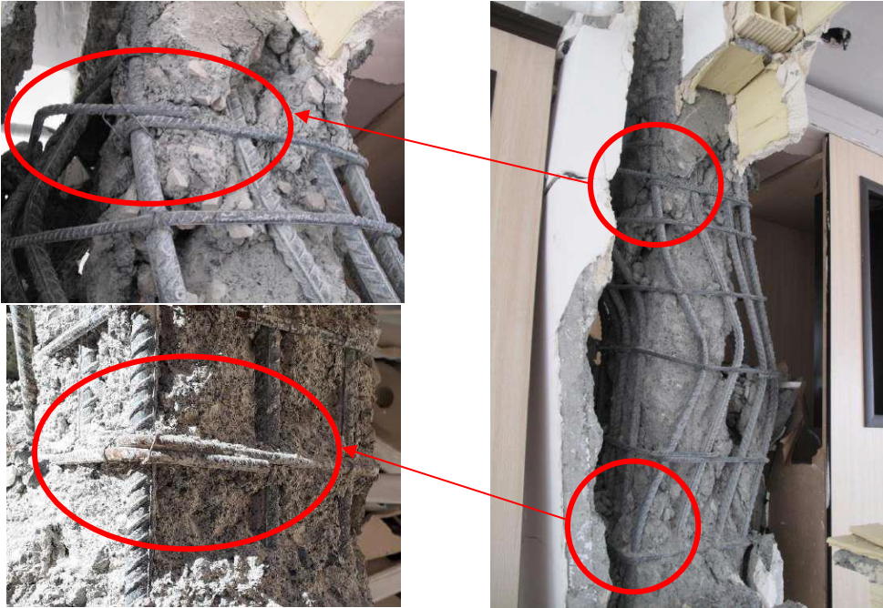
Figure 10. Inadequate anchorage detail in column
