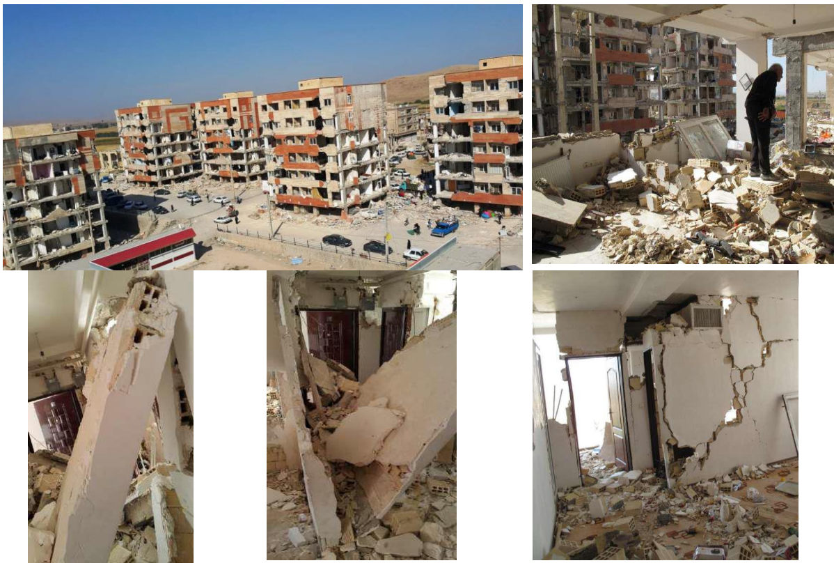
Figure 12. Collapse of facade, infill panel and non-structural walls of Shirodi development.
