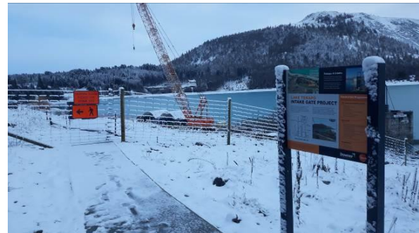
Figure 2: Extreme temperatures were a risk to concrete quality
