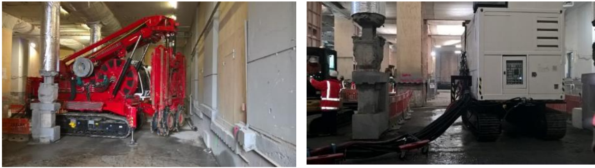
Figure 4: Hydrofraise D-wall machine (left). D-wall Power Pack detached (right). The Hydrofraise compact was the only machine capable of constructing the D-walls inside the building and was the first time this equipment was used in New Zealand
