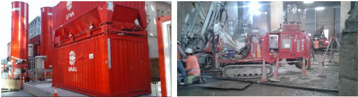
Figure 6: Bentonite D-wall and jet grout plant (left) Jet Grout Piling Machine (right)
