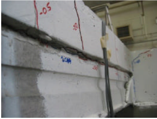
(a) Delamination of the topping concrete
