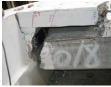
(a) North side failure
