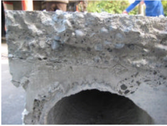
(c) Hairline crack showing some delamination of the topping.
