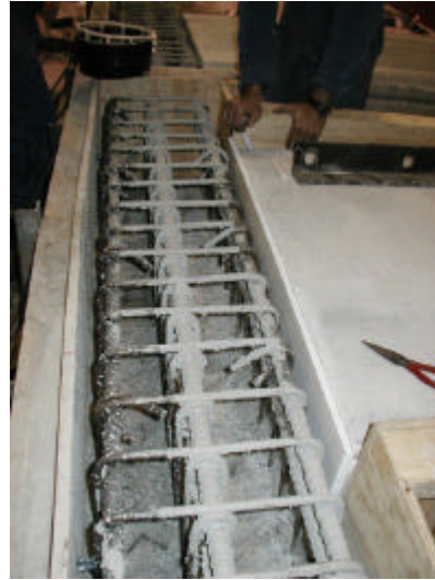
(b) Unit in place before starters are attached
