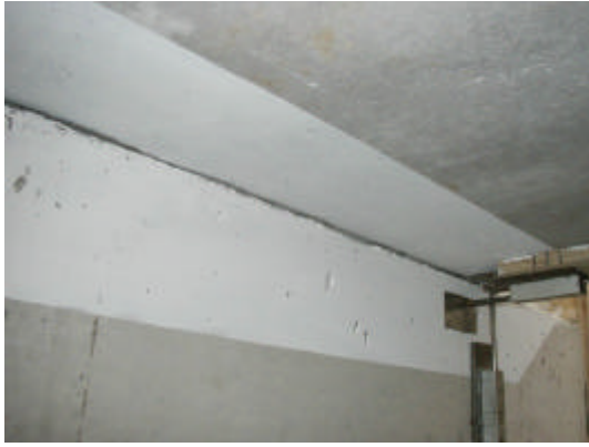
(a) Sliding of the hollowcore unit relative to the supporting beam.
