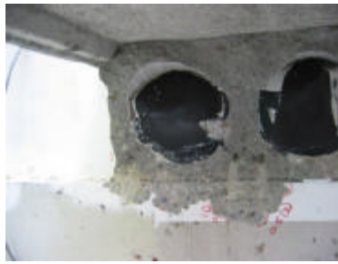
(d) A photo showing when the prestressing strands pulled out of the end of the hollowcore unit
