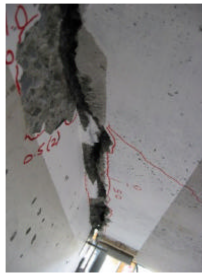
(b) Dropping of the hollowcore unit and damage to its seat.
