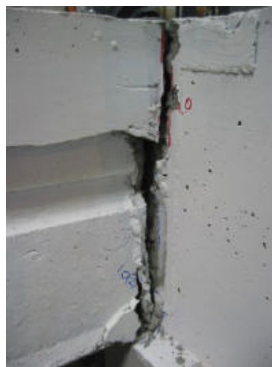
(b) Side elevation of the fracture
