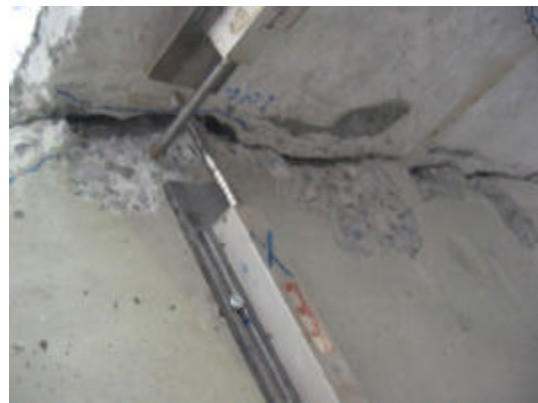
(b) Damage to the underside of the hollowcore unit
