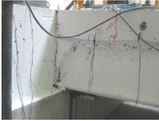
(a) Seat damage at 2.0% (1.62%) drift
