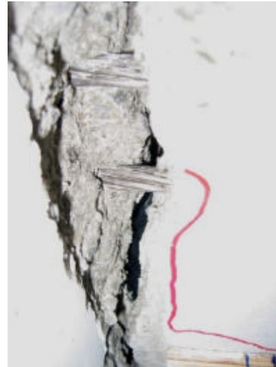
(a) The crack was large enough to pass a ruler through the gap between the unit and the beam. (b) The prestressing strands pulling out of the fractured hollowcore unit.
