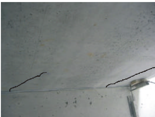
(a) Longitudinal cracks in the bottom of the hollowcore unit (Drift= 1.0\% ( 0.58\% ))
