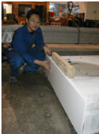
Figure 3-6. The compressible backing board placed on the end of the hollowcore unit.
