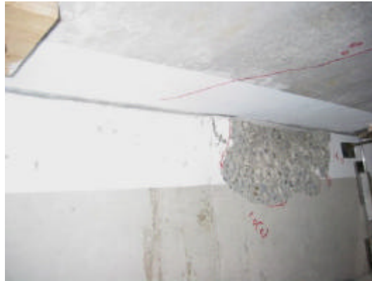
Figure 5-14. Spalling of the beam cover concrete (Drift=1.0%).
