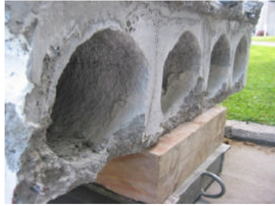
(d) The very bottom of the hollowcore unit fractured.
