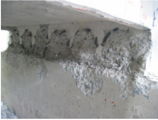
(c) Damaged seat.
