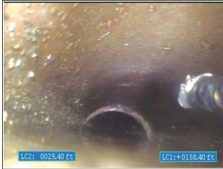
Figure 6—Example of water at the base of the interior of a sewer lateral as viewed by an inspection crew's camera.
