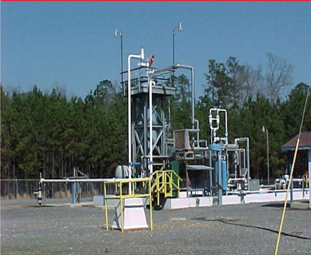
Typical Brine Supply Well
