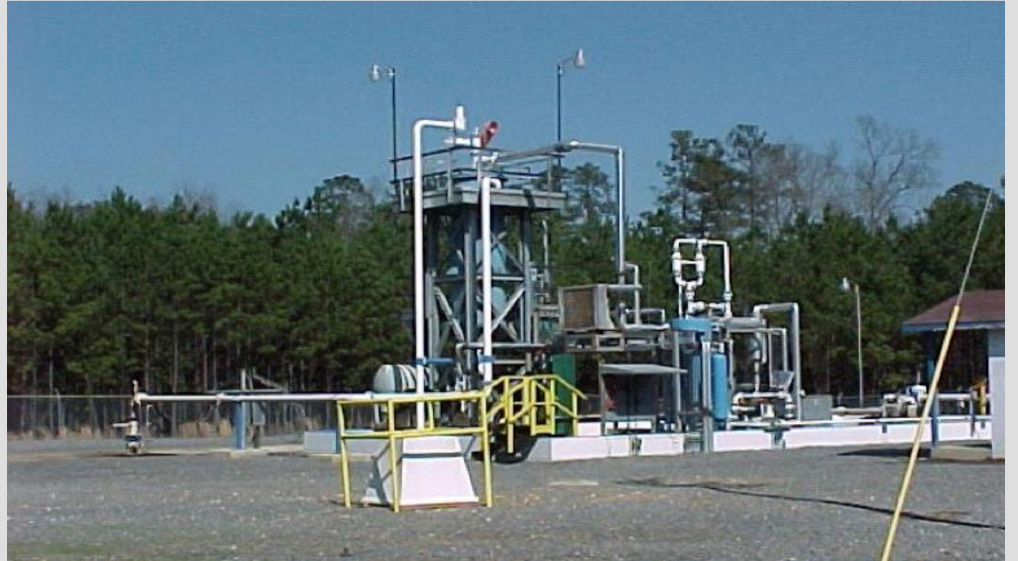
Typical Brine Supply Well
