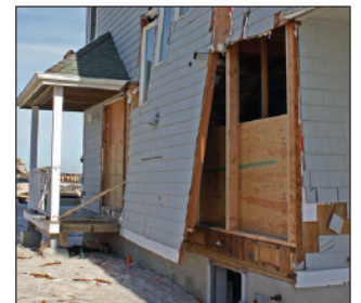
Figure 1: Back wall failure due to flood level above the lowest floor of a house in Ortley Beach, NJ.
