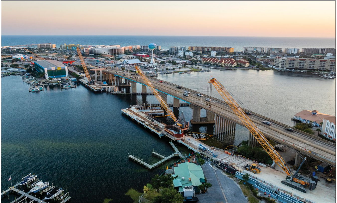
Aerial view of the Brooks Bridge project in Santa Rosa Sound between Fort Walton Beach and Okaloosa Island. The new bridge will vastly improve traffic flow between the two communities. Photo courtesy of Superior Construction.
