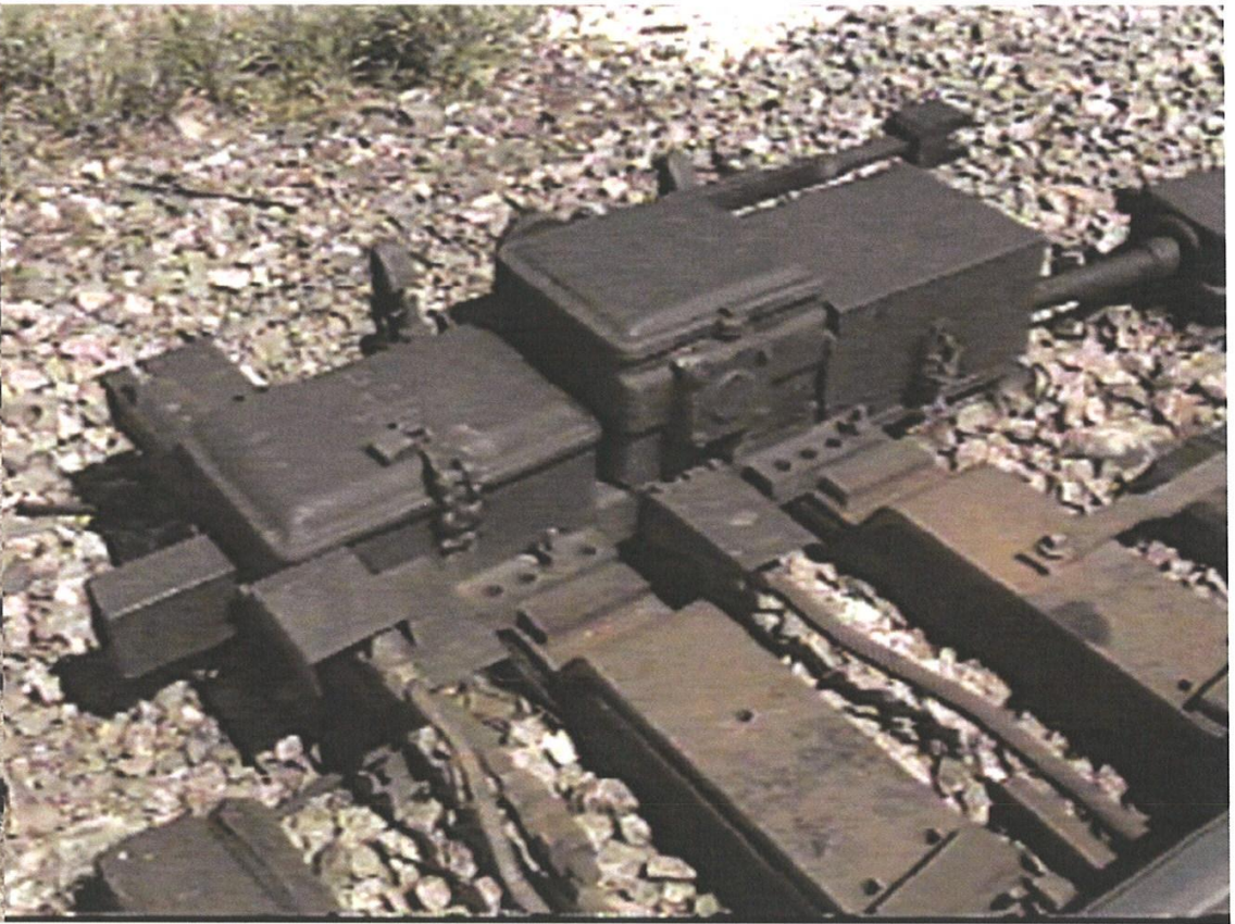
Figure 3-31 Dual Control Switch Machine – Photo by J. E. Riley
