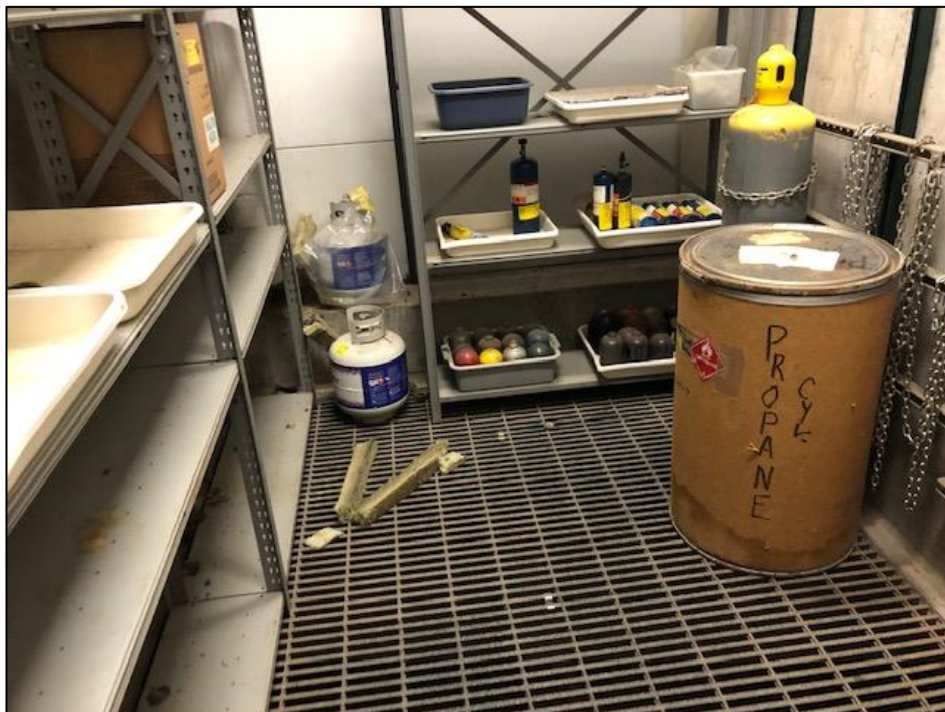
FIGURE 9: TCEM 118 Damage (insulation)
