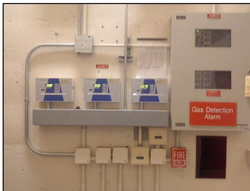
Figure 2 – Gas Detection Alarm System
