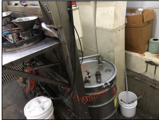
Figure 1 – Grounding/Bonding of Transfer Drum
