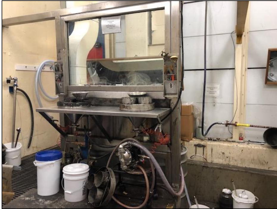
FIGURE 2: TCEM 117 Flammable Liquid Processing Station
