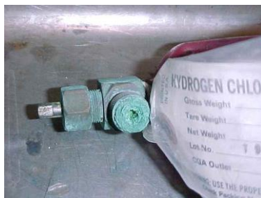
Corroded valve on a hydrogen chloride lecture bottle.
