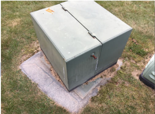
The picture above shows the result of a pad-mounted transformer that was struck by a riding lawnmower.
