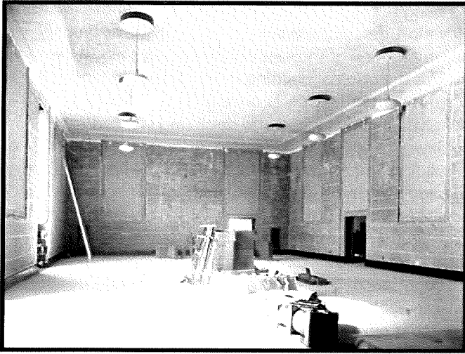
In a photo from 1934, construction continues on the West Ceremonial Courtroom of the courthouse in Mobile. (National Archives at Atlanta)
