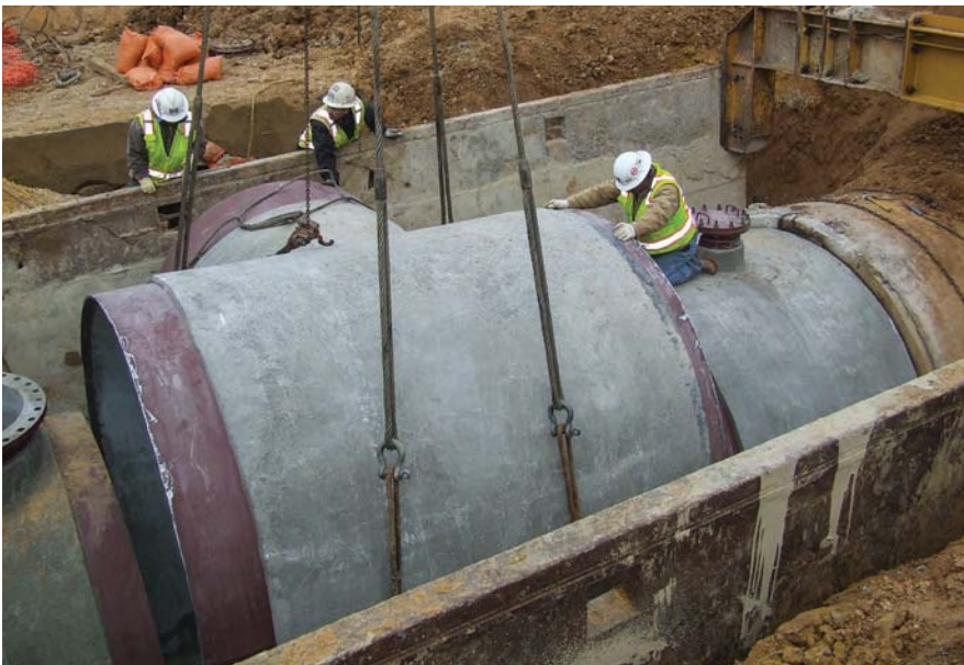
A key sustainable component was the use of native controlled low-strength material (CLSM), rather than gravel, for pipeline embedment. Field testing was used to evaluate the feasibility of CLSM; numerous sample pits, pictured, were filled with mixes of different soil types and different proportions of cement content.
