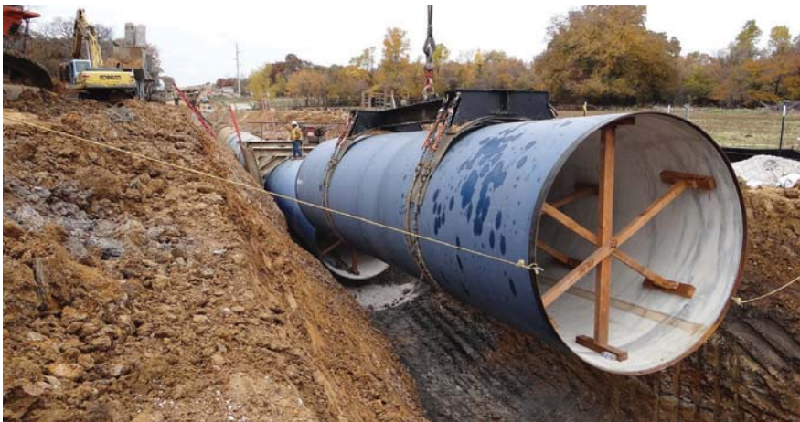
Stulls were installed inside the pipe to maintain its shape and protect its lining during delivery, storage and installation.
