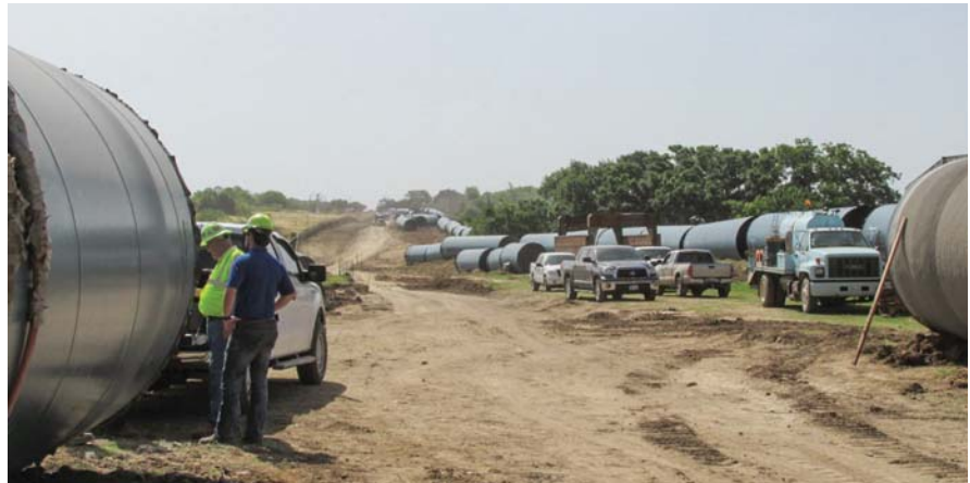
The world's first Envision-rated pipeline is the Line J, Section 1 Pipeline, a 2-mile segment of the Tarrant Regional Water District raw water delivery system in Texas. It received an Envision Silver Award in 2014.
