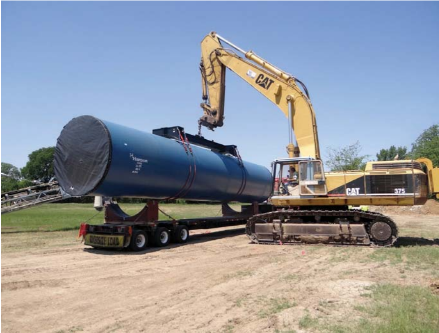
Line J is made up of 108-inch-diameter steel pipe. Two processes that were evaluated for triple-bottom-line impact were the manufacturing of the pipe, and its transportation to the project site from four different plants across the United States.
