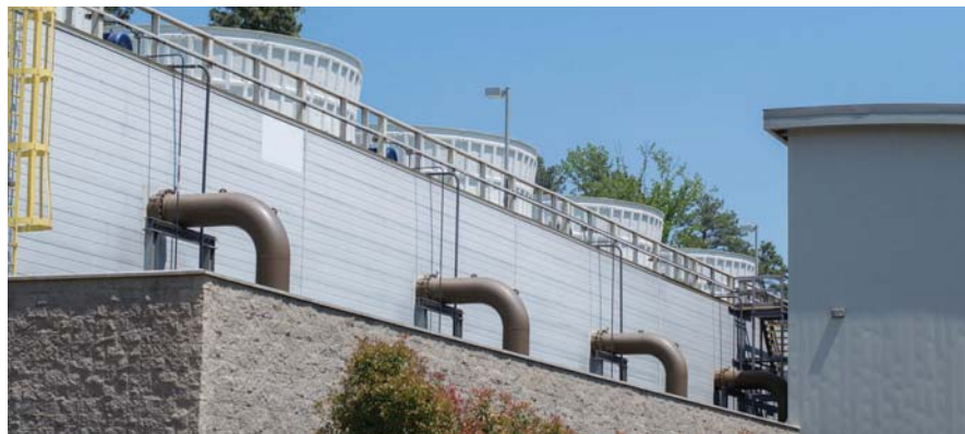
Chiller Plant #2 cooling towers
