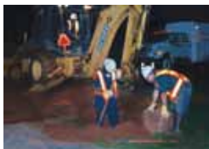
Utilities is a 24/7 operation. Maintenance and construction crews repair an average of 2 leaks per crew per day.
