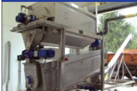
DSP Screw Press Model 3012, NY WWTP
