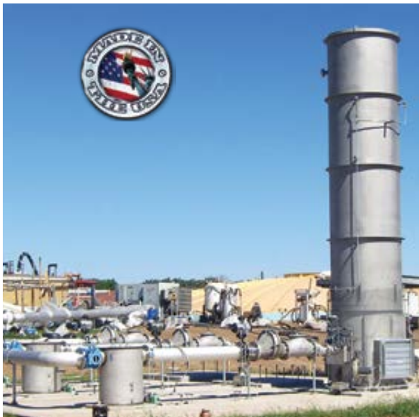
Enclosed Burner with Remote Tip Ignition
