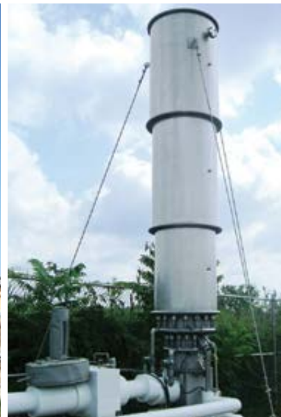
Enclosed Burner with Ground Level Ignition Remote
