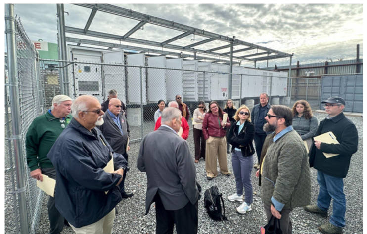
Site tour with local officials at a 5 MW energy storage facility in Brooklyn, developed and operated by Microgrid Networks.
