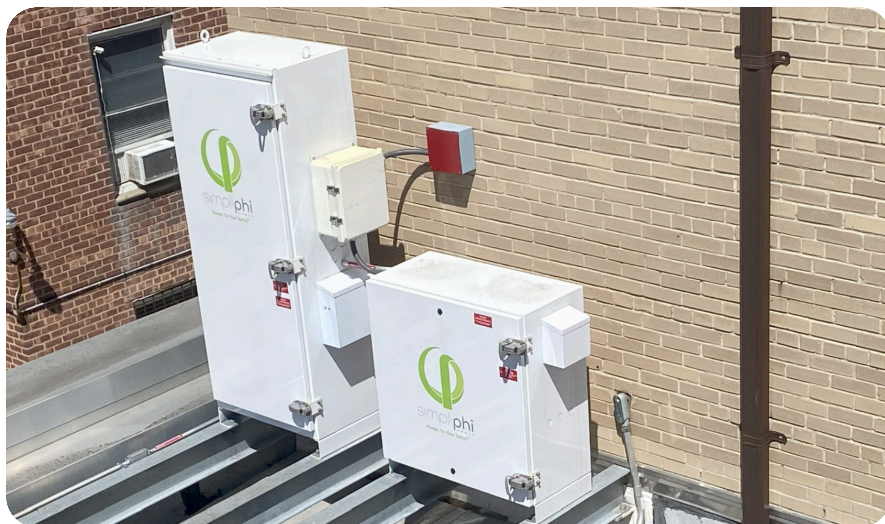
This 19 kWh Simpliphi battery was installed alongside solar panels on the rooftop of the Kings Highway branch of the Brooklyn Public Library. The system provides energy bill savings and backup power. The project was a collaboration between Accord Power, Solar One, the New York City Department of Citywide Administrative Services (DCAS), and the Governor's Office of Storm Recovery (GOSR). Courtesy of Accord Power.
