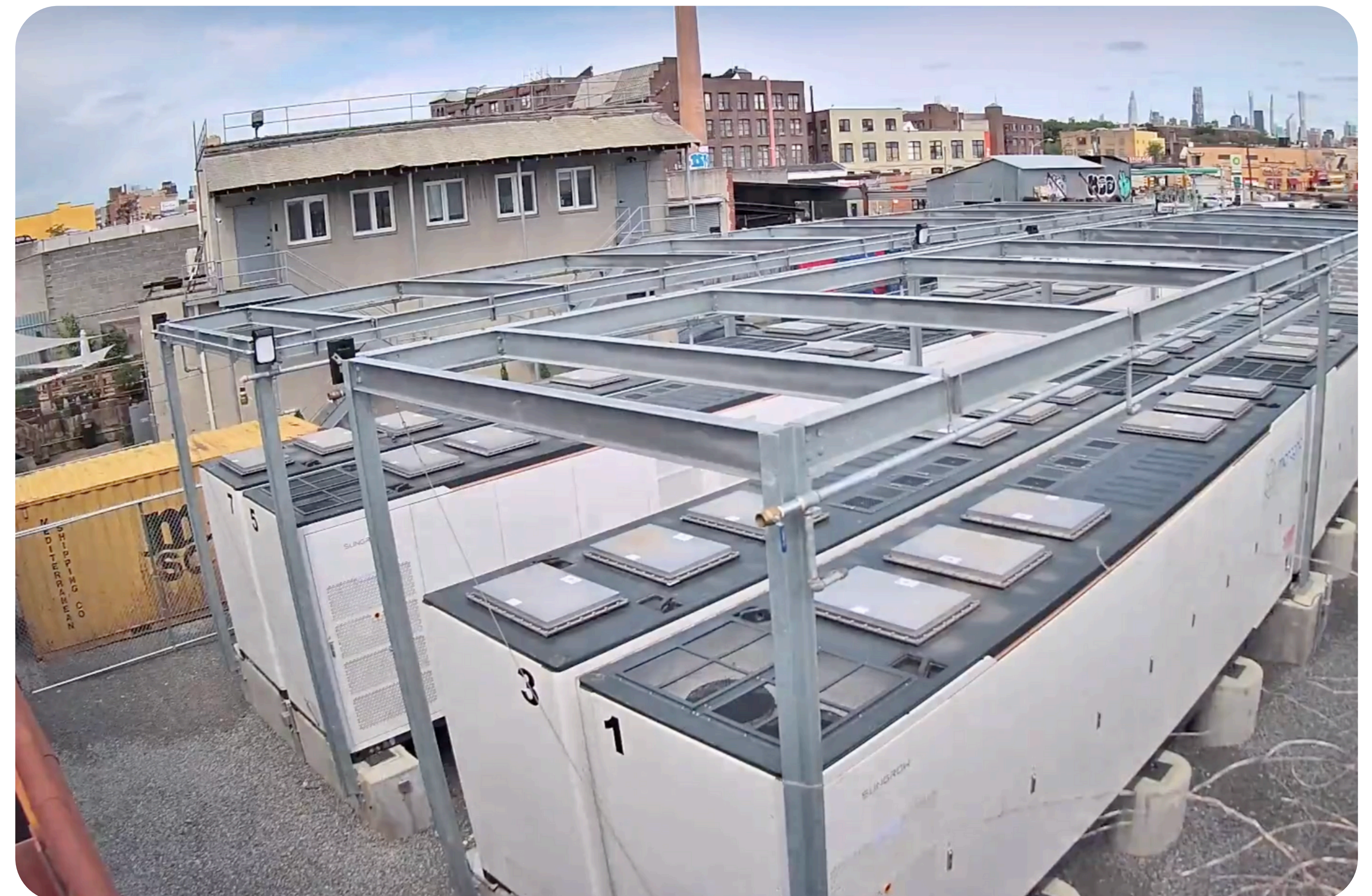
5 MW energy storage system installed by Microgrid Networks, providing grid services to Williamsburg, Brooklyn. Courtesy of Microgrid Networks.
