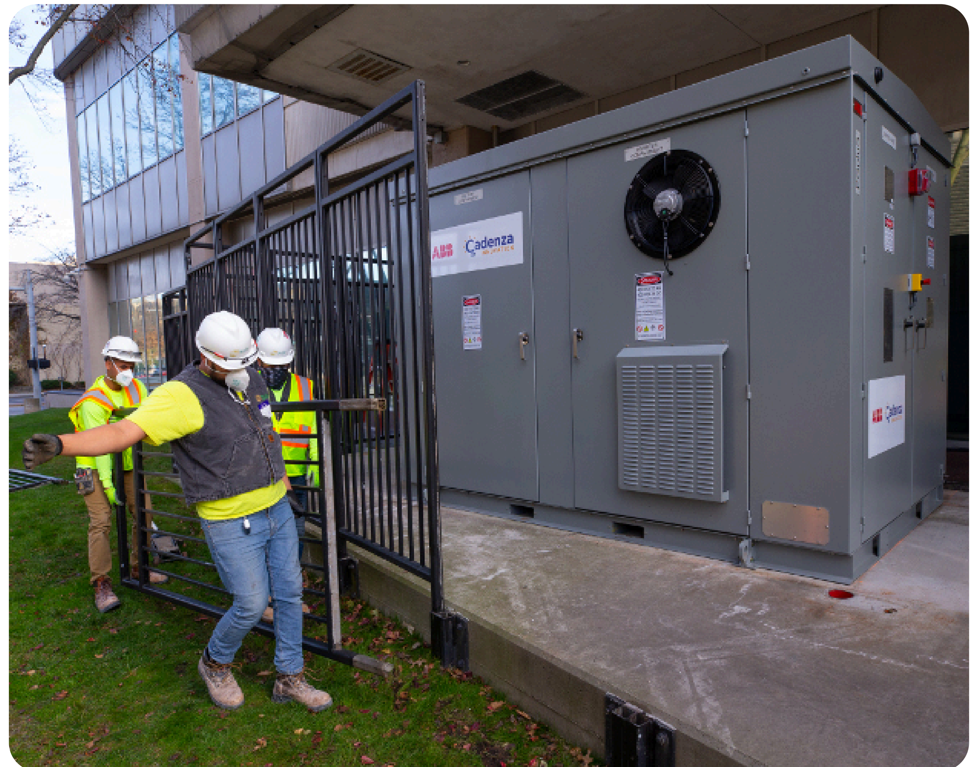
A 50kW / 250kWh Cadenza Innovation battery that provides peak-shaving services and bill reductions for the New York Power Authority (NYPA) headquarters in White Plains, New York. The project was partially funded by a grant from the New York State Energy Research and Development Authority (NYSERDA). Courtesy of Cadenza Innovation.
