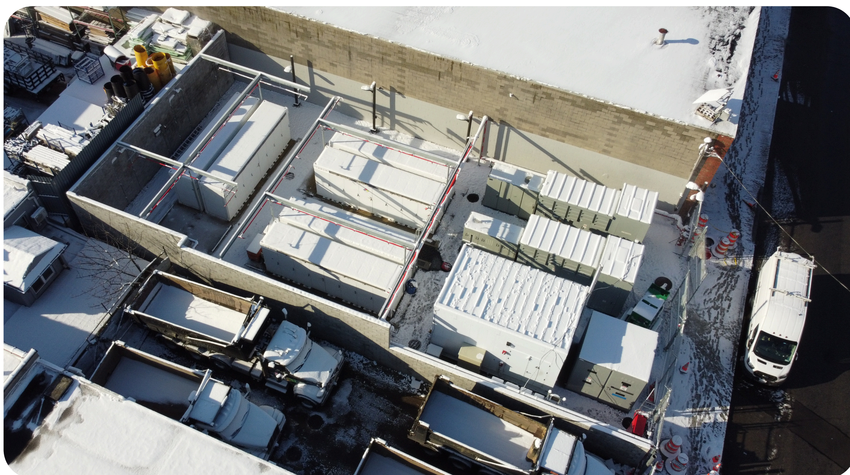
Birds-eye view of a 5 MW energy storage system installed by Soltage, providing grid services to Maspeth, Queens. Courtesy of Soltage.
