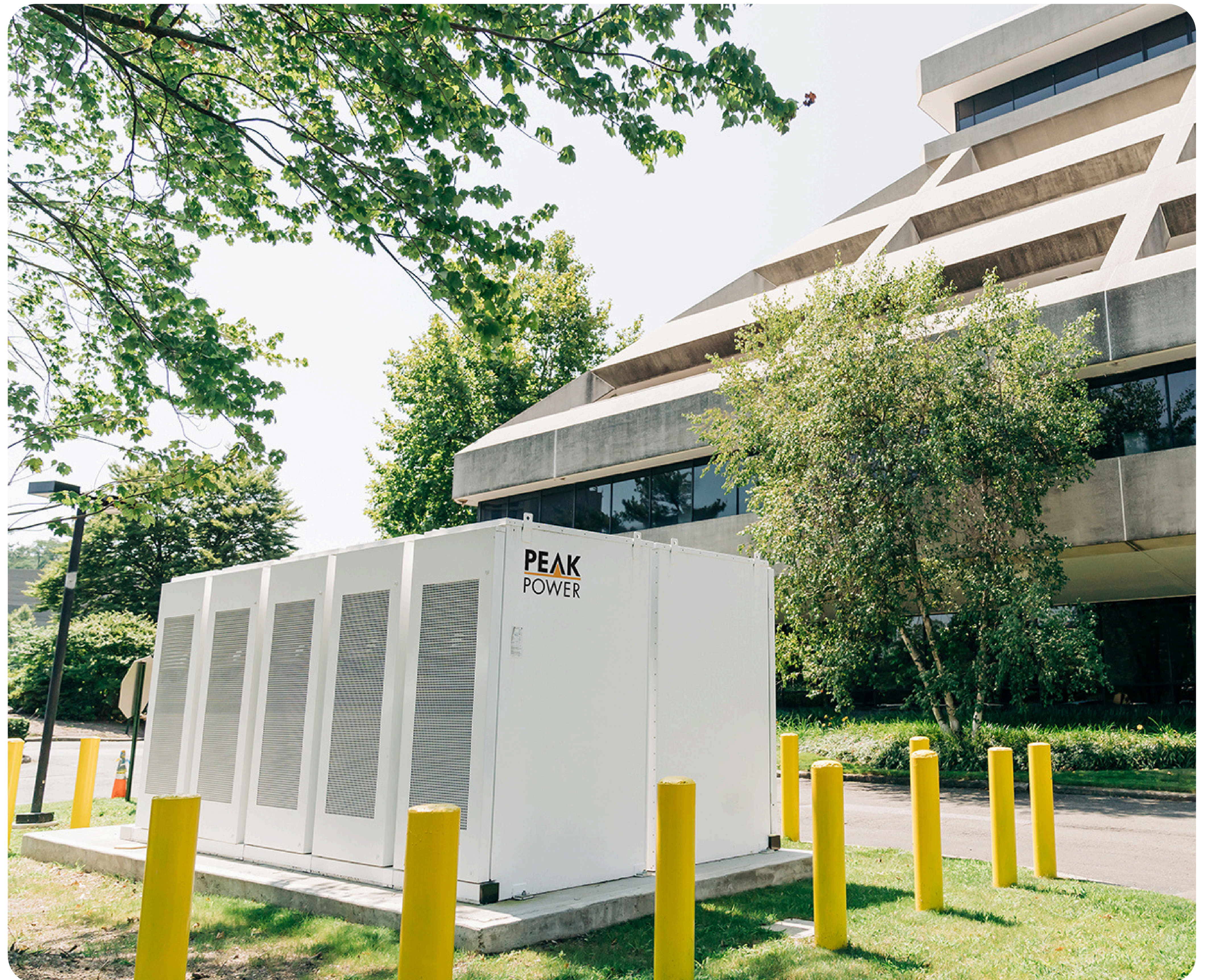
One of four battery systems installed by Peak Power in a commercial office complex in Westchester, New York. Collectively, the systems provide 1,334 kW / 5,336 kWh of energy storage capacity and represent one of the state’s first Virtual Power Plant demonstration projects. The project reduces electricity costs and participates in NYISO and ConEd demand response programs. Courtesy of Peak Power Battery Storage.
