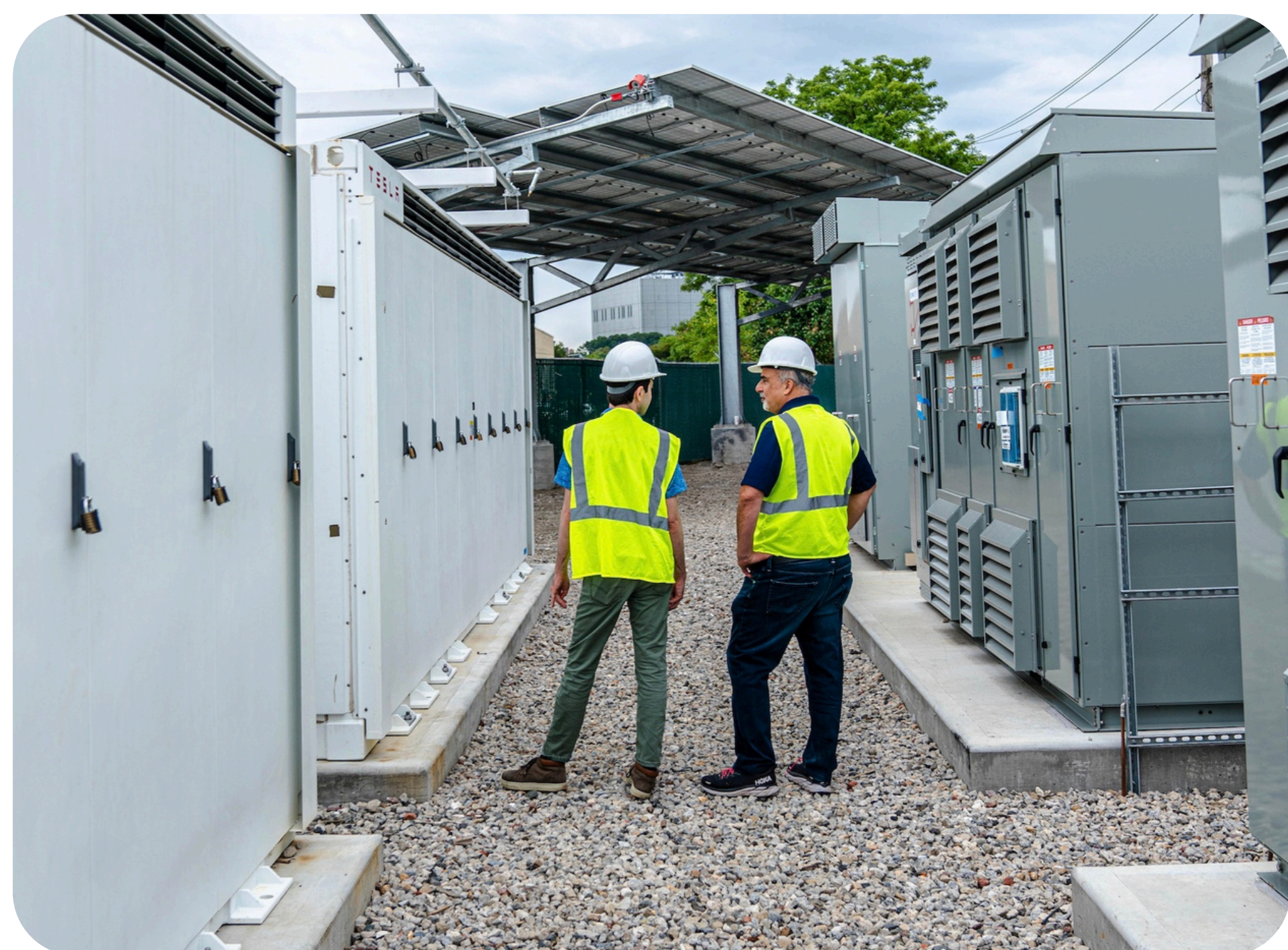
3 MW community battery project built by NineDot Energy, providing grid services to the Pelham Gardens neighborhood of the Bronx. Courtesy of NineDot Energy.
