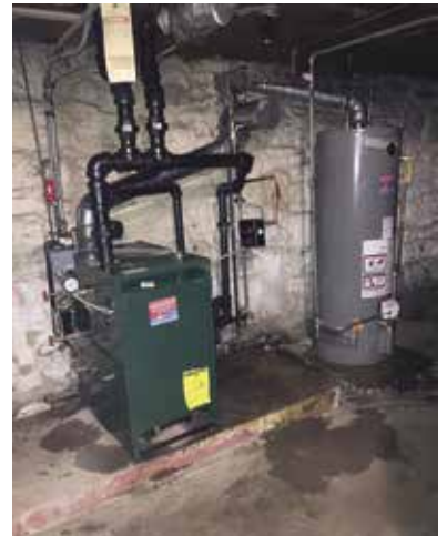
New boiler & water heater
