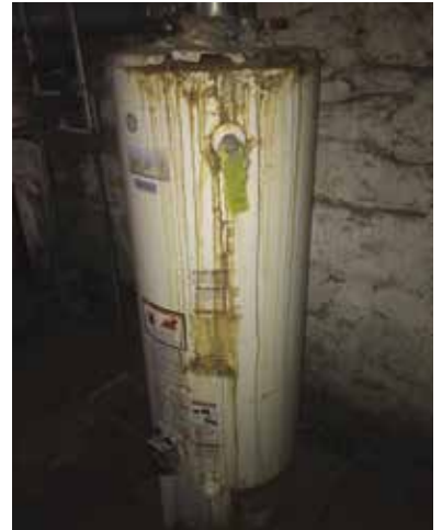
Old water heater
