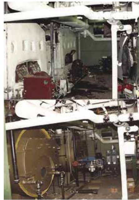
McCready & Rice Boiler Plant
