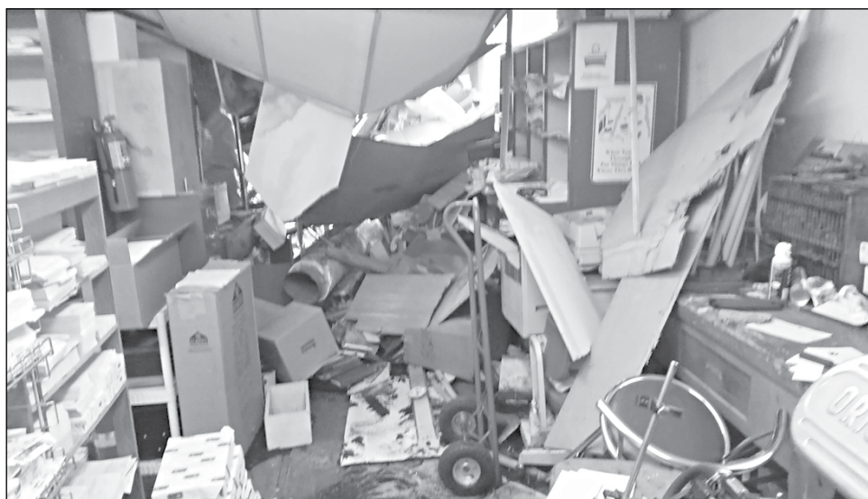
Rusty Ferguson, publisher of The Cleveland American, broke the news of the collapsed ceiling at The Cleveland American on Facebook, along with photos of the damage.
