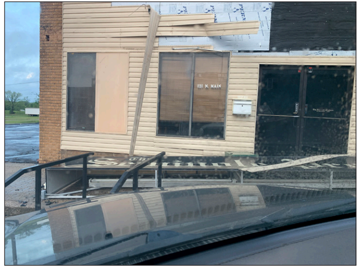
The Seminole Producer's office received extensive damage in the May 4 tornado. The newspaper's signage was pulled off the building and siding peeled away. Many businesses in downtown Seminole were damaged in the storm.
