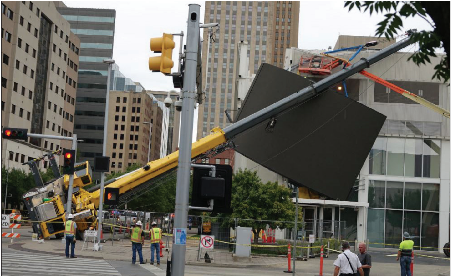
Crews inspect a crane that fell into the side of a building in downtown Oklahoma City at Robinson and Sheridan avenues.
