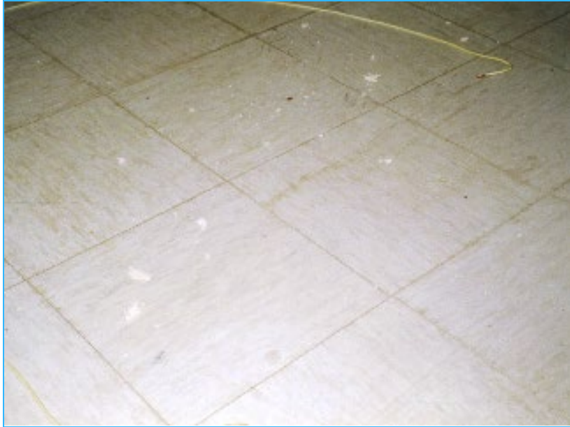
Vinyl Asbestos Tile
