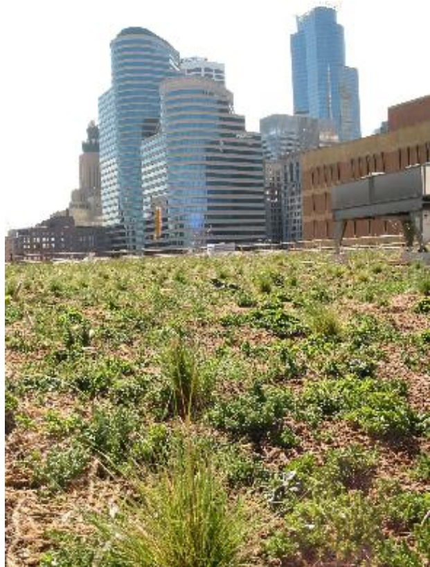
Minneapolis Central Library Green Roof. Image courtesy The Kestrel Design Group, Inc.
