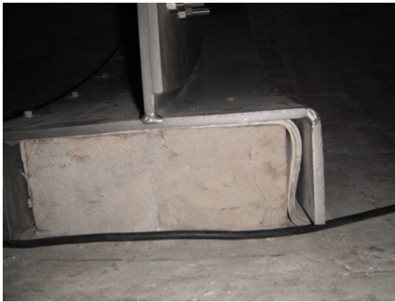
Pueblo Viejo AUT-150: Compartment call anchored by corbel brick. Ceramic paper installed for relief of thermal expansion.
