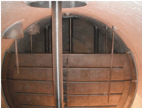
Pueblo Viejo AUT-150: Compartment 4 wall with compartment wall baffle installed (at centre).
