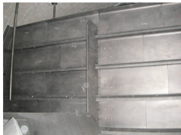
Pueblo Viejo AUT-150: Reverse (discharge) side of compartment 3 wall. 'C' channels, stiffener rings and wall baffle.
