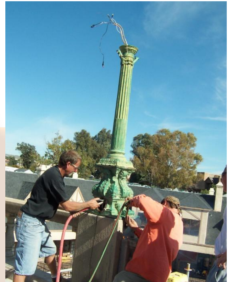
Removed lamp post to find why stone was cracking
