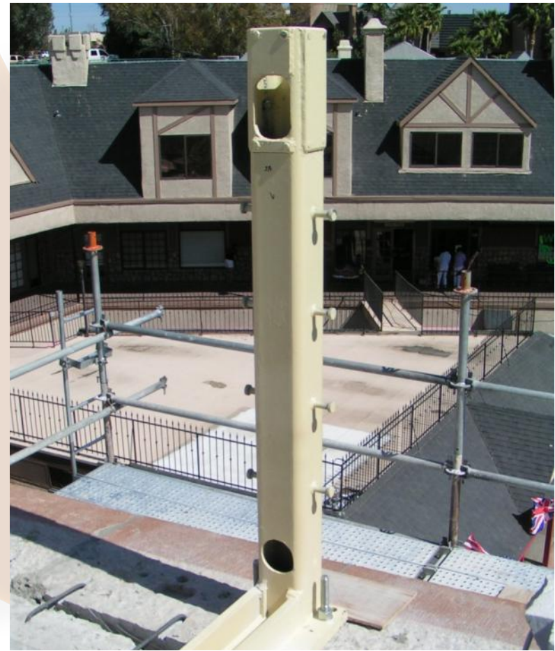
Replaced existing rusted lamp support post with new epoxy coated steel post
