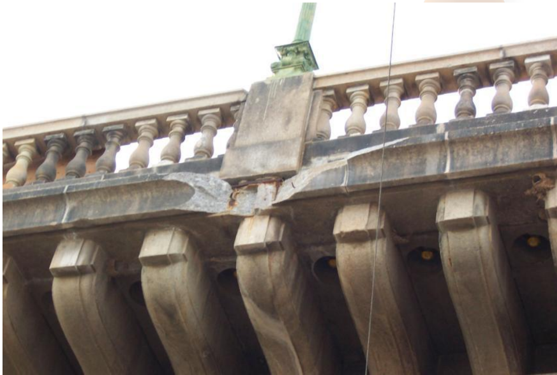
Coping stone cracking at each lamp post
