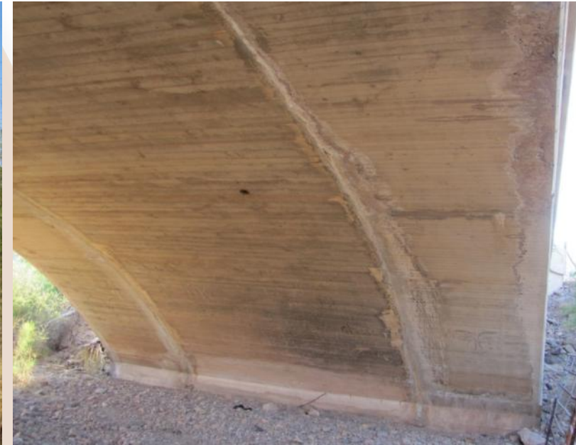
Lowell Arch Bridge remains in use by widening the bridge rather than replacing it.
