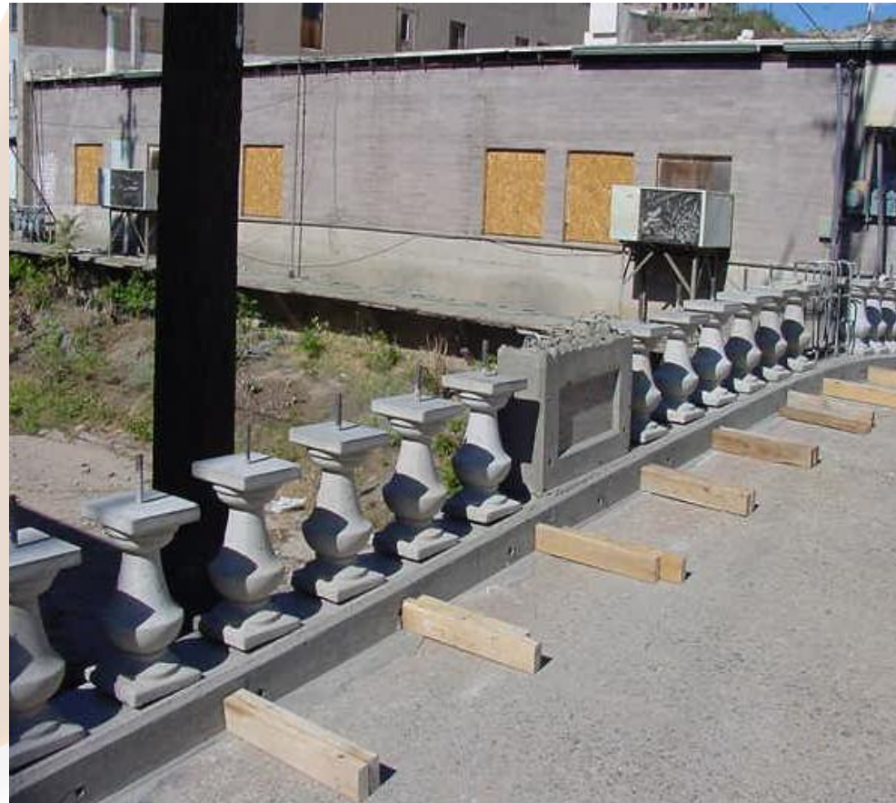
Replaced barrier rail with near replica of Historic railing. Precast balusters in place and ready for placement of concrete top rail.
