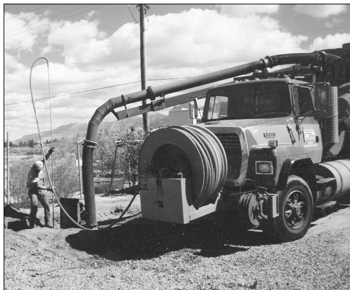
Front view of vacuum truck and operator pre-wetting soil with pressurized water hose for soil removal by vacuum hose on right side of operator.
