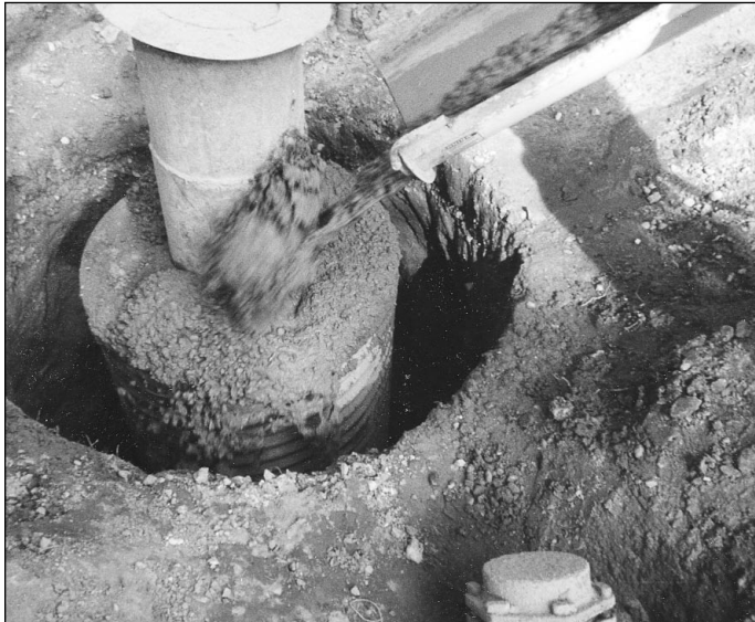
Close up of cement grout being added to annular space. Fine and coarse grain texture of alluvial deposits can be seen in hole profile.
