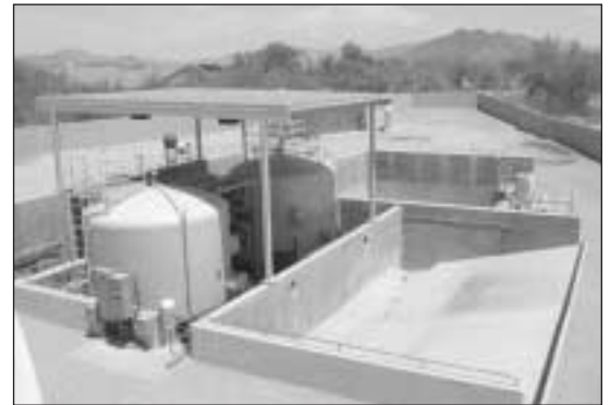
Figure 1- COP Arsenic Treatment Facility at Well 280
